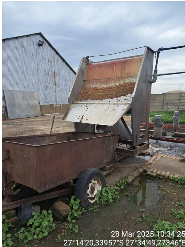
Photo 07: Waste water treatment facility
